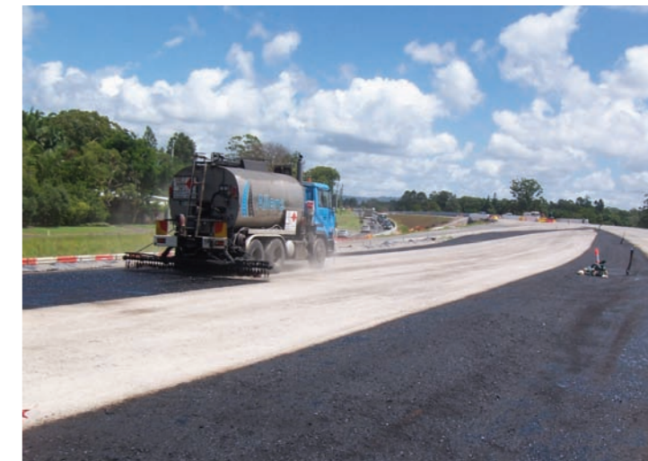
Priming of final layer of pavement prior to sealing and asphalt works
